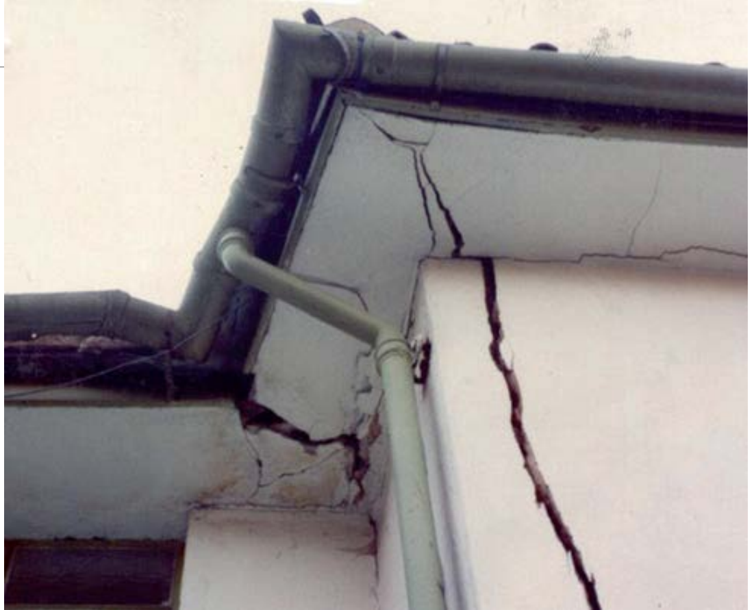
Structural damage to house caused by “end lift” (by Peter Kelsey & Partners)
